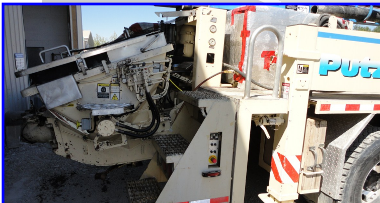
Figure 3 Back Hopper to Putzmeister Piston Pump system
