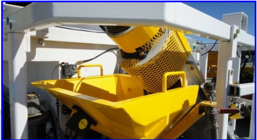
Figure 7 Mixing Auger Discharge to Aliva 257 hopper
