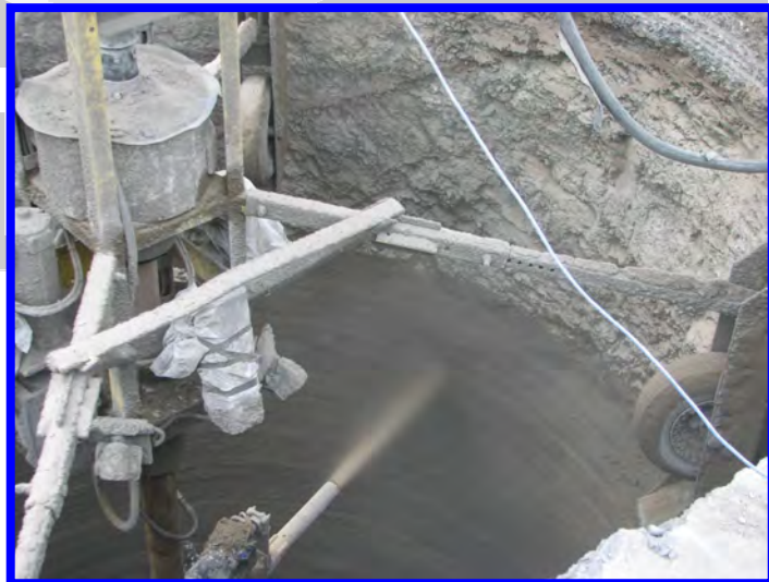
Multicrete Raise Robot™ Completing Top Meter of 3.5 m x 300 m Deep Raise
